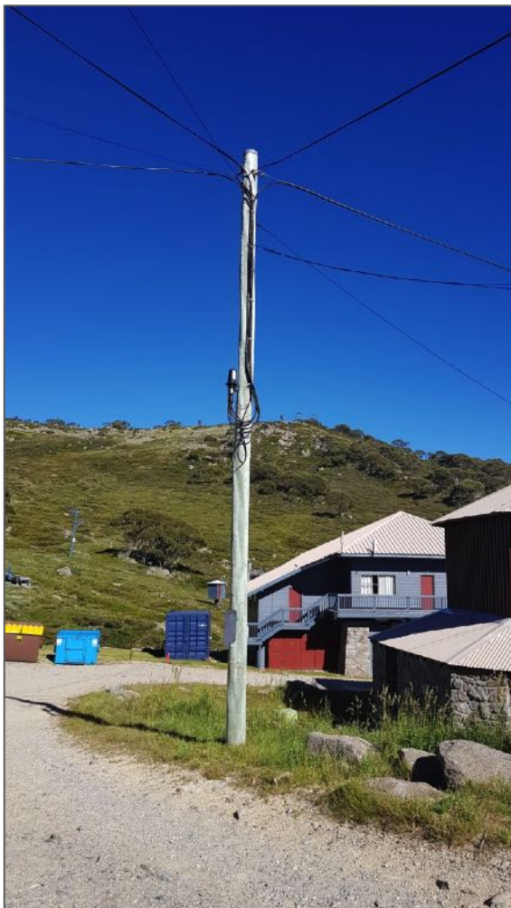
Figure 6. Timber utility pole
